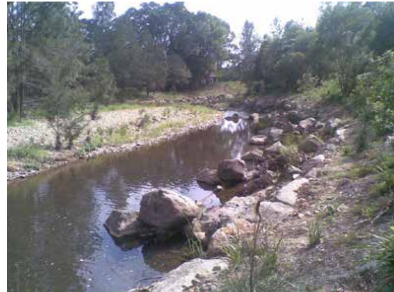
Currumbin Creek: Post restoration works Bank toe reinforced with LWD & rock scallops. Reveg establishing behind structure.
