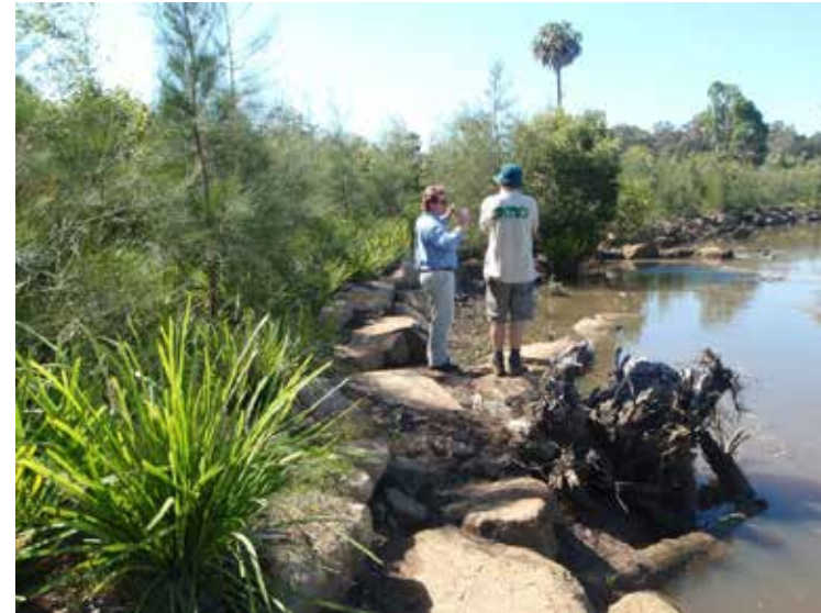
Post restoration works 27-10-10: Bank toe reinforced with LWD & rock scallops. Mangroves & reveg establishing behind structure.
