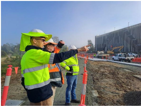
Project Manager, Peter Van Esseveld tours the site with John Ryan, Department for Transport & Main Roads
