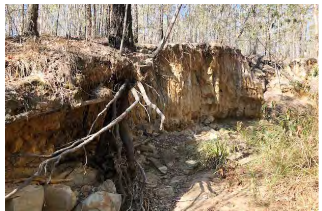
An estate waterway with eroded creek bank
